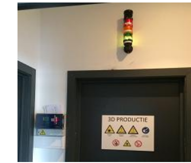
Safety installation at the entrance of a customer lab
